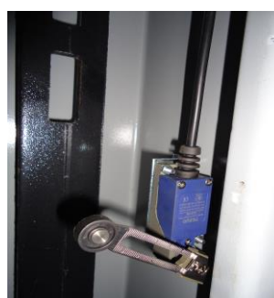
Picture 19 (Lower limit switch)
